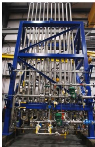
Figure 3 IsoFlo™ Black Liquor Oxidizer, pipeline reactor
