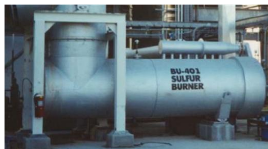
Figure 3 Installed sulphur burner
