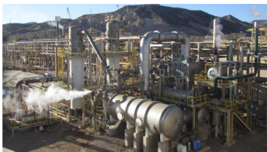
Figure 2 NORAM SO 2 plant
